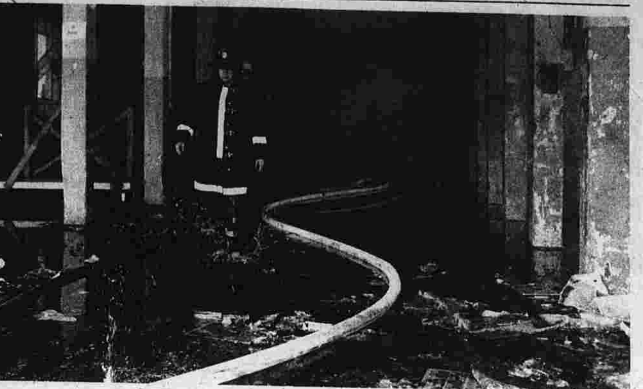
Warehouse Damaged by Fire A member of the Eighth District Fire Department checks lines at a fire yesterday afternoon at a warehouse on Hilliard St. The fire was controlled quickly by firemen and the building's sprinkler system. Cause of the fire is under investigation. (Herald photo by Dunn)
